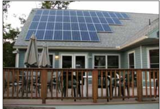
Solar Panels on common house at Pathways Cohousing, Northampton, MA.
